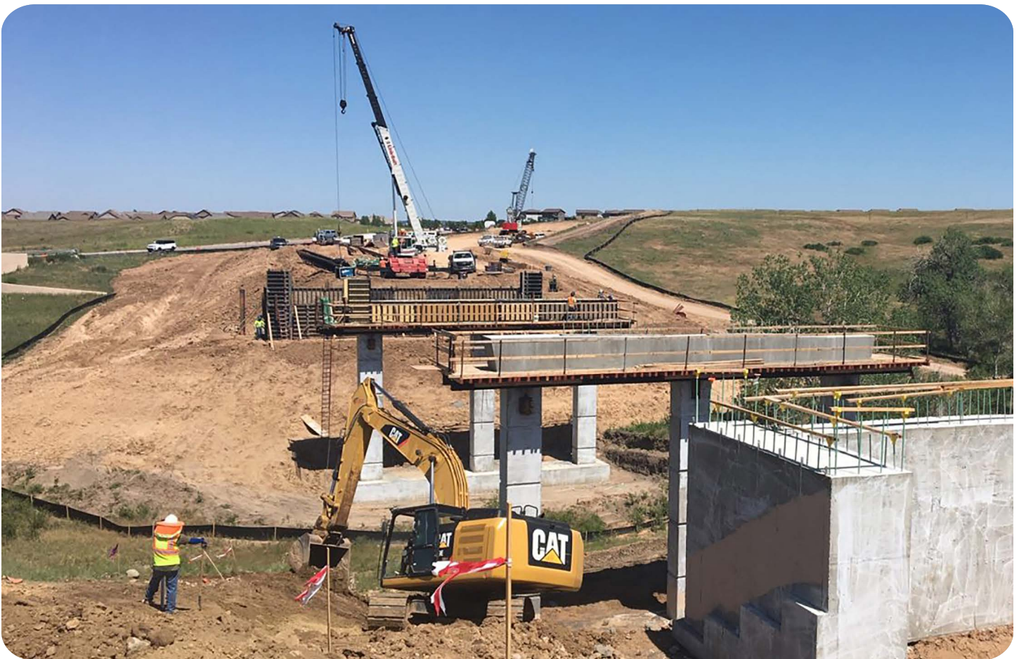
Of the 3,116 bridges in the Denver region, 45 are considered to be in poor condition. Maintenance and reconstruction activities improve the quality of bridges throughout the region, including along RidgeGate Parkway in Lone Tree. Photo courtesy of the City of Lone Tree.
